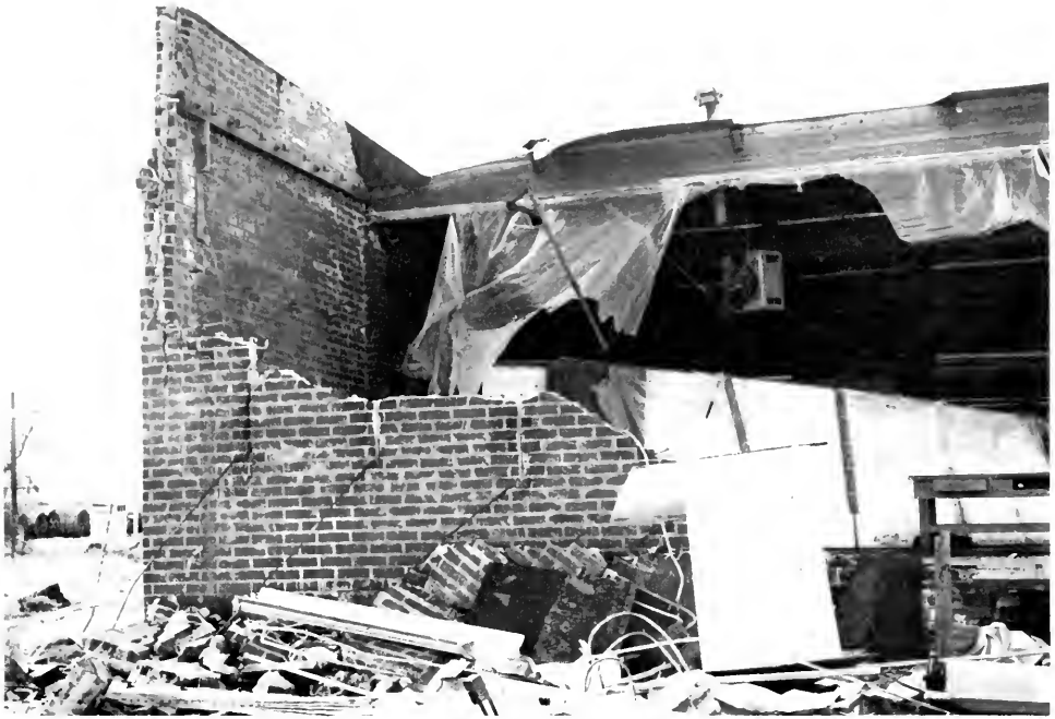
Photo 21. Masonry structure, as noted in this picture, generally sustained greater damage than wood frame structures.
